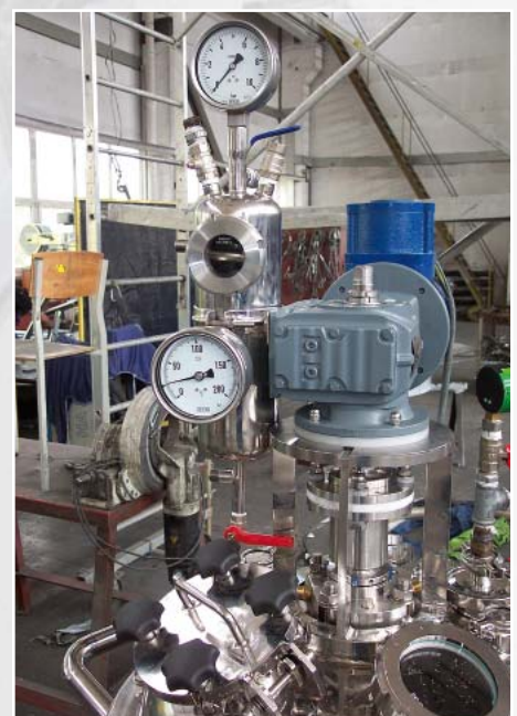
A mechanical seal auxiliary system
