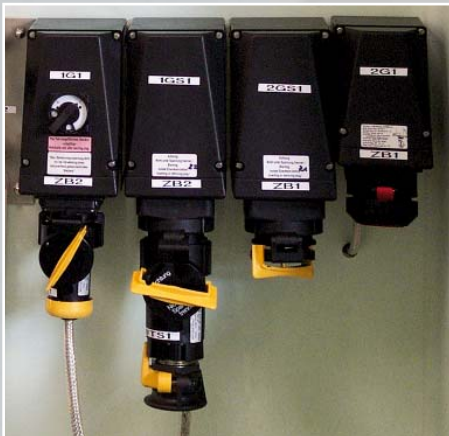
An electrical terminals assembly in the zone
